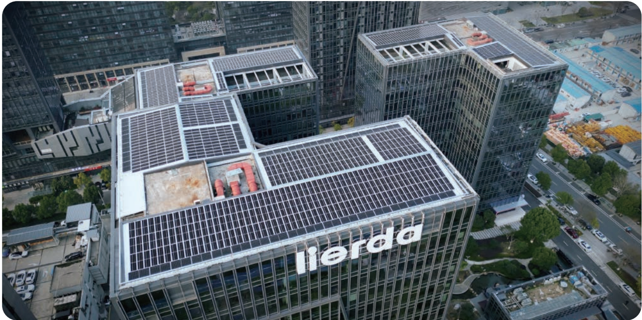
265KW Location: Zhejiang, China Date of installation: 2024 Project type: C&I - BIPV
