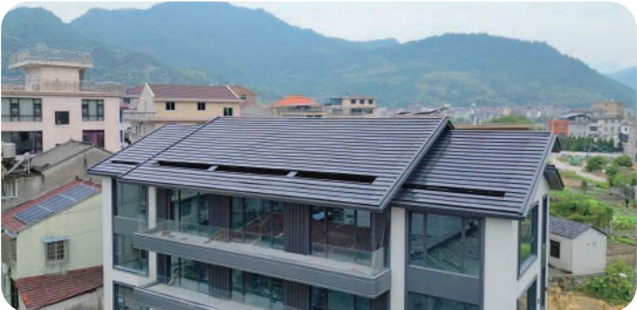
35KW Location: Zhejiang, China Date of installation: 2023 Project type: Residential - BIPV
